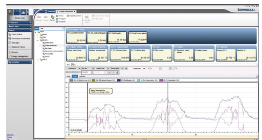
brewmaxx EnMS is fully integrated in the user interface of the process control system.
